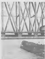
THE HUGE pipe still tower was floated by barge to the refinery site.
